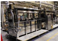
Cooling system for care food production
